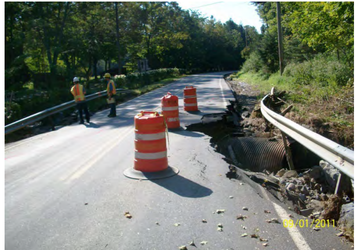
FIGURE 5. DAMAGED ROAD AND CULVERT AFTER TROPICAL STORM IRENE IN 2011. PHOTO SOURCE: DCTC
