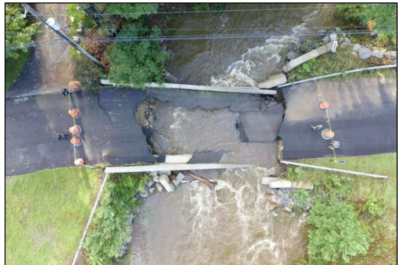
FIGURE 2. BRIDGE WASHED AWAY AFTER HURRICANE IDA FLOODING. PHOTO SOURCE: DAILY VOICE.
