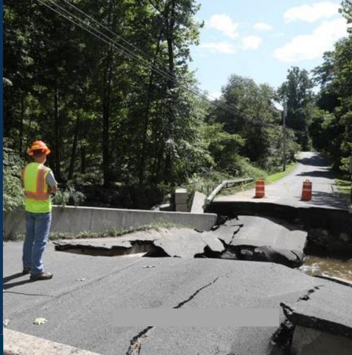
Bridge over Wicopee Creek, East Hook Road (Tropical Storm Ida)
