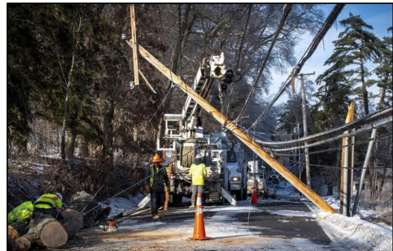
Figure 14. Central Hudson repairing a damaged utility pole blocking the road following a winter storm (Source: Central Hudson)
