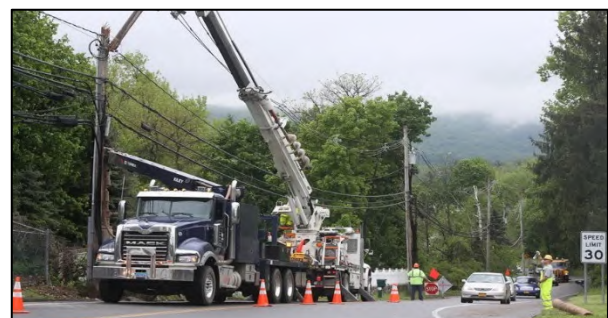
Figure 16. Central Hudson replacing a damaged utility pole following a severe storm (Source: Poughkeepsie Journal )
