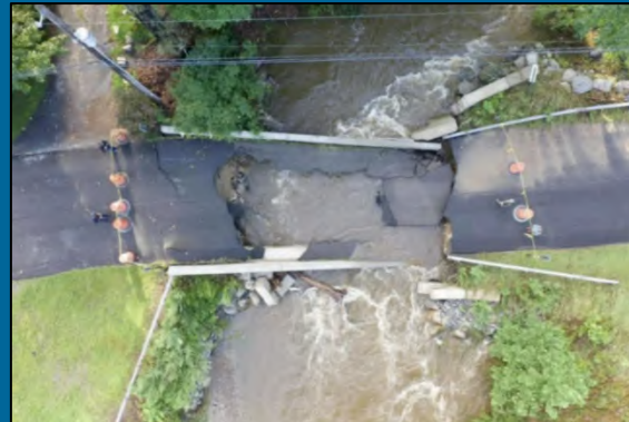
During Hurricane Ida in 2021, 4-6 inches of rain fell overnight, washing out a large culvert. A State of Emergency was issued for the entire county.
