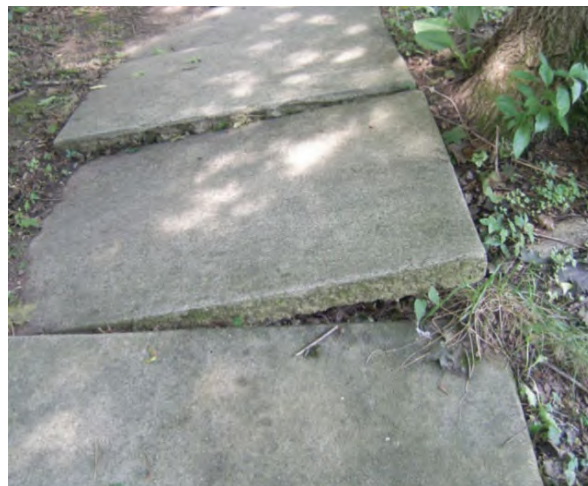
Figure 41. Sidewalk being lifted due to tree root interference (Source: DCTC )
