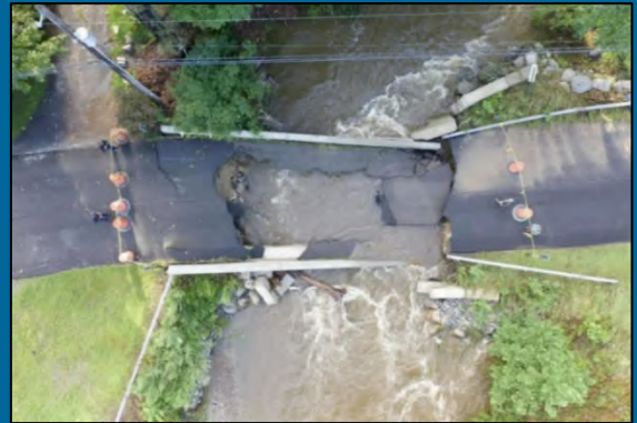
During Hurricane Ida in 2021, 4-6 inches of rain fell overnight, washing out a large culvert. A State of Emergency was issued for the entire county.
